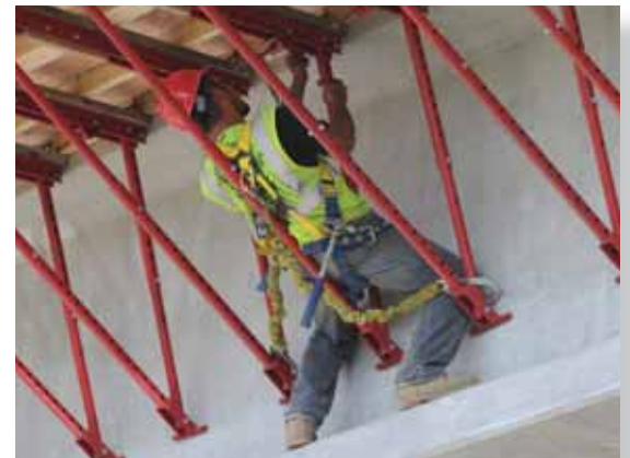
Bridge inspector examines high beam on the I-29 Overpass at 52nd Avenue South in Fargo, North Dakota. Photo courtesy of Terry Wiklund, North Dakota Department of Transportation, 2008.
